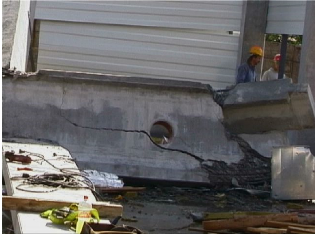
Destruction of a concrete truss, photo: Prof. Radim Cajka
